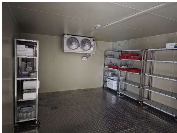
Cold room (refrigerator)
